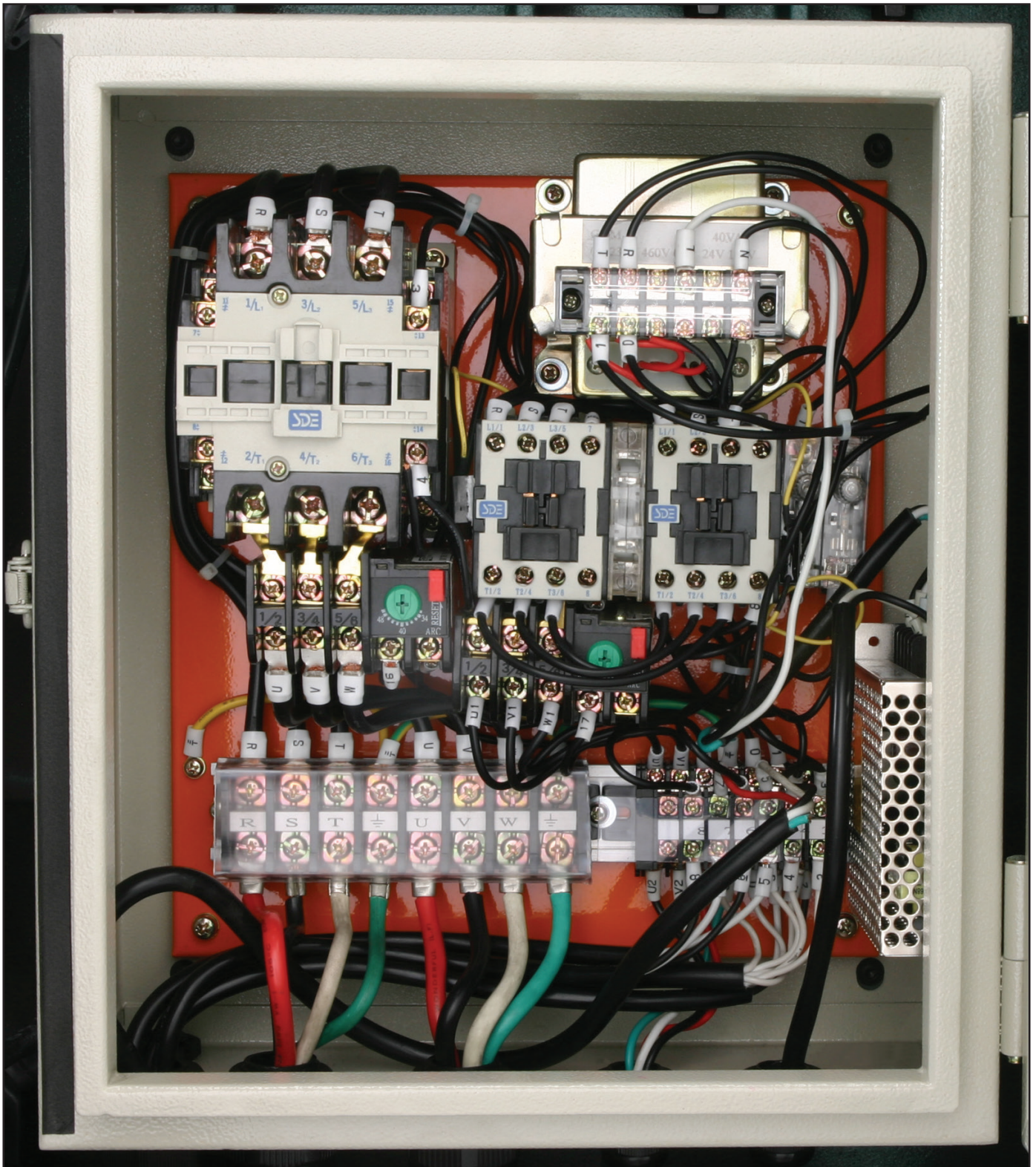
Figure 50. Main electrical box (top right access panel removed).
