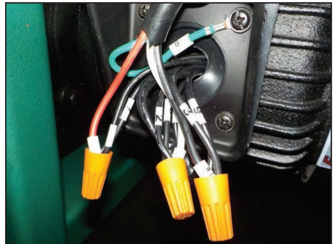
Figure 55. Table motor junction box wiring.
