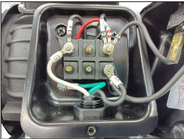
Figure 107. Motor junction box wiring.
