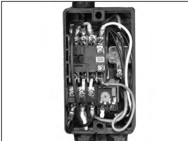
Figure 4. 220V Magnetic Switch
