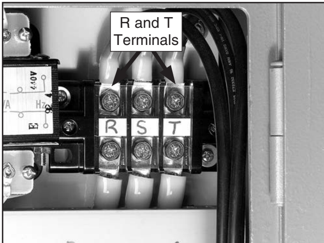
Figure 22. Close-up view of power supply terminals inside electrical panel.
