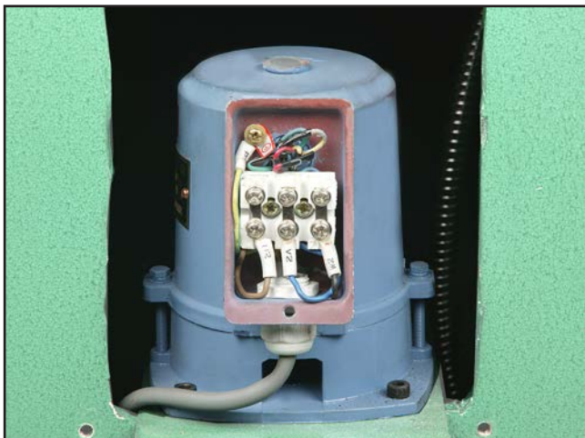
Figure 78. Pump motor (M2) connections.
