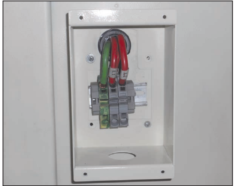
Figure 78. G0449 power junction box.
