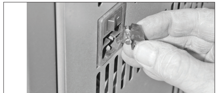
Figure 20b: Main power switch
