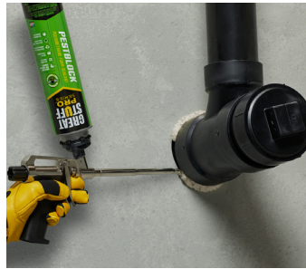
PVC pipe penetrations
