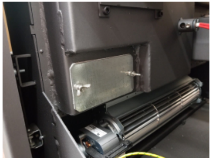
Figure 33A: Exhaust Chamber Cover Plate. Air Intake side
